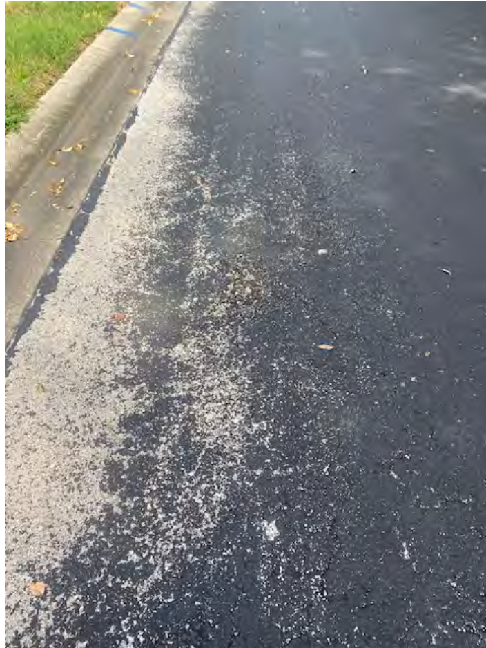
Figure No. 4. Raveling and Cracking Conditions Observed on Rosehaven Drive.
