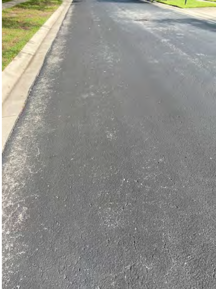
Figure No. 1. Cracking Condition Observed on Amberside Way.
