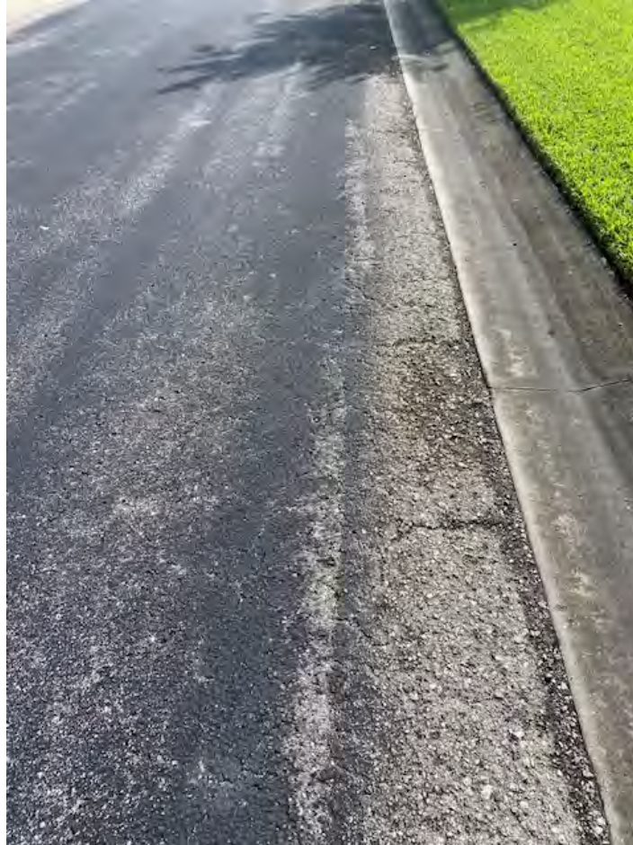
Figure 3. Raveling Condition Observed on Rose Haven Drive.
