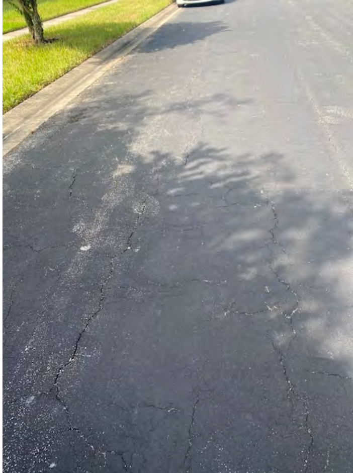
Figure 2. Cracking Condition Observed on Spring Hollow Loop.
